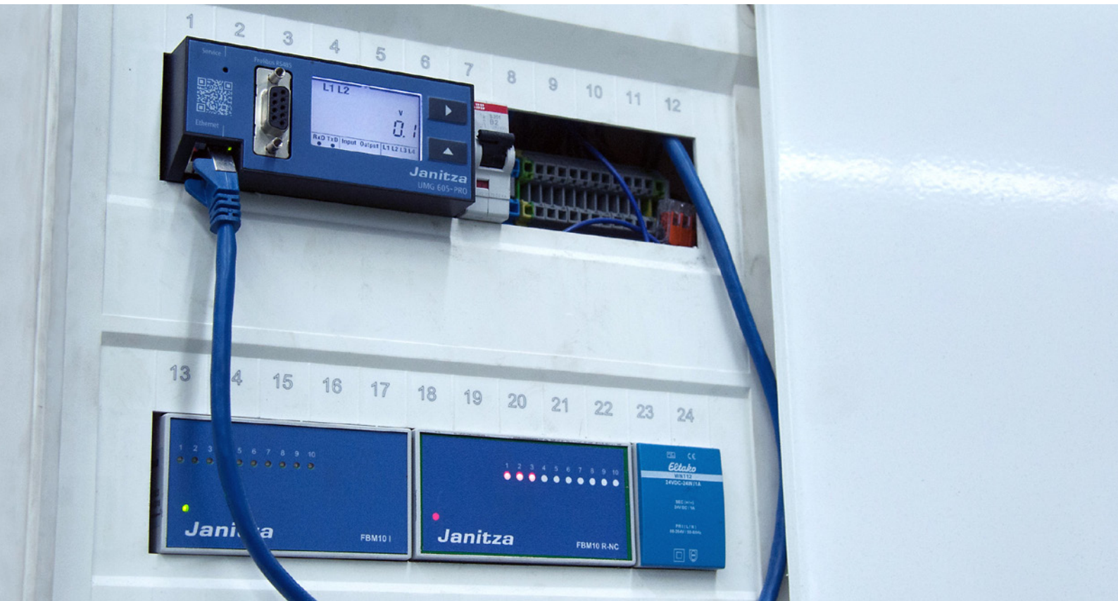
The Janitza UMG 605-PRO network analyzer obtains the synchronization pulse directly from the energy supplier's electricity meter.
